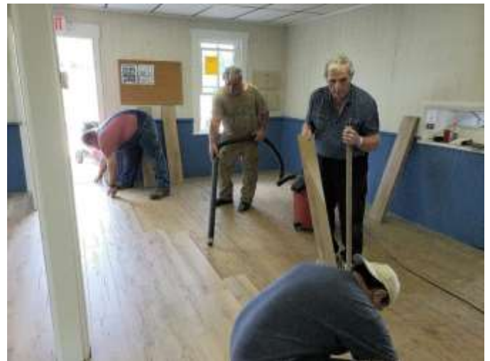
The new flooring project took about 15 hours – all accomplished in one day by volunteers!
